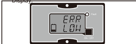
5. Battery low volt protection.
